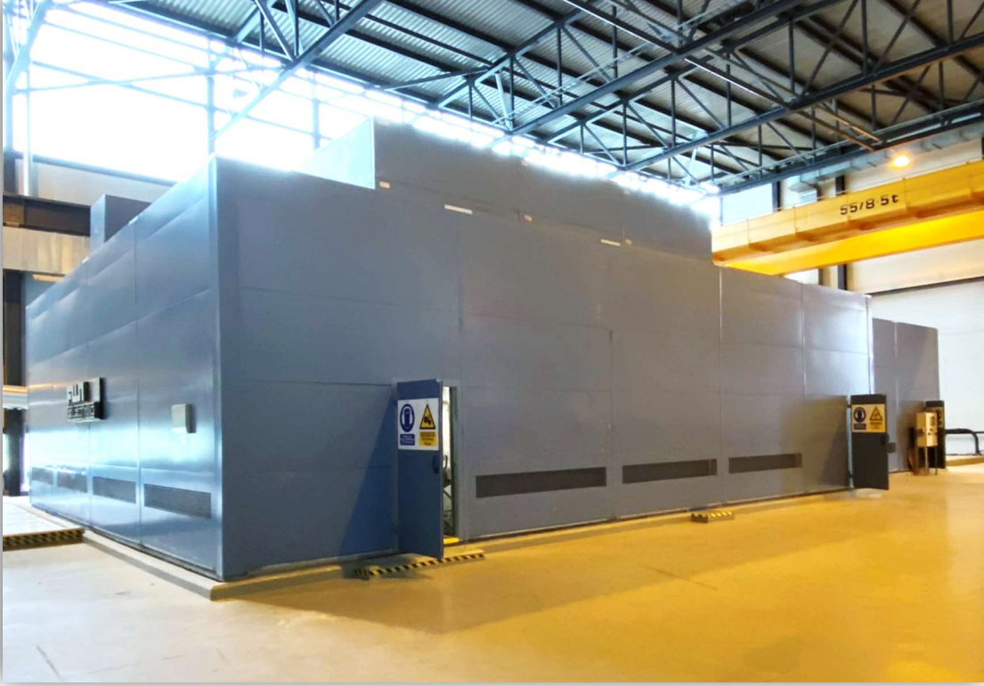
plant inside view – steam turbine / power generator set
